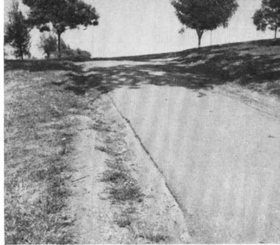
Water was encouraged to run off to the sides of this path, causing the erosion shown along the edge.
