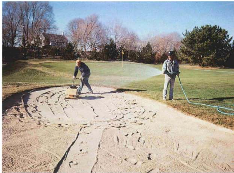
The application of water to the newly installed sand produces an ideal base on which the cement finisher can move.
