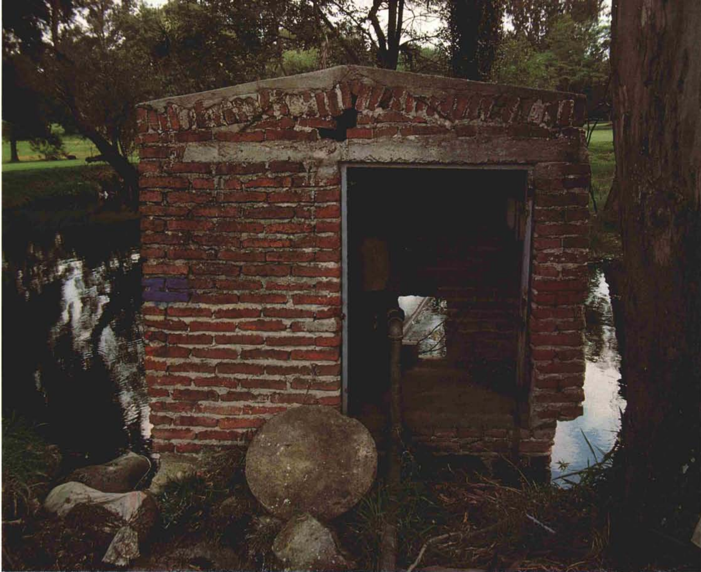
High-voltage hazards should be secured.
