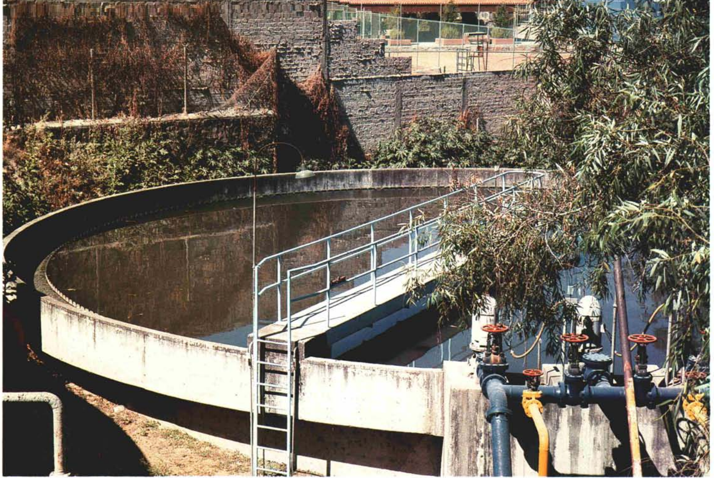
To produce usable effluent for golf course irrigation, the water is screened and treated.
