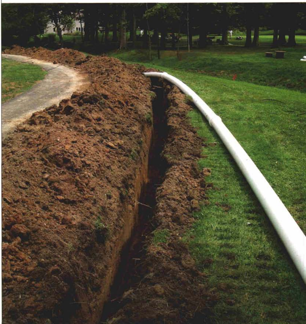
A topnotch new automatic irrigation system with good control and hydraulic flow is an essential tool for effective water management.
