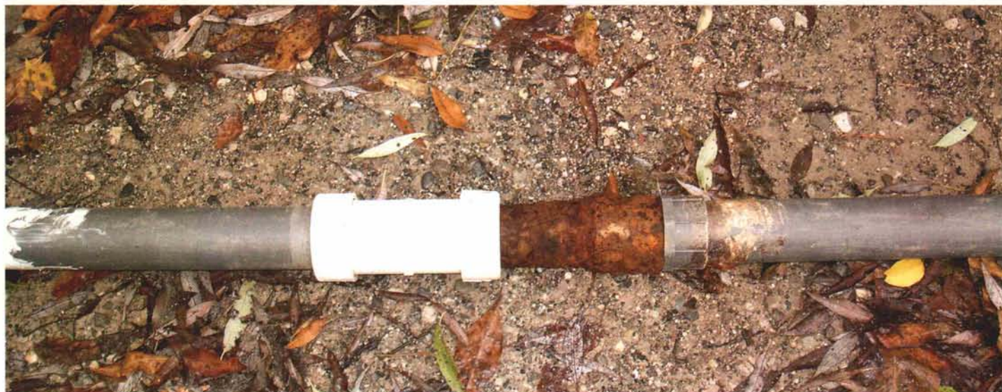
Corroded old pipes were no longer capable of providing adequate hydraulic flow, so coverage and turf performance suffered.
