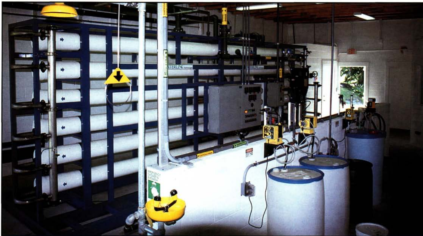
The filtration vessels are at the heart of the reverse osmosis water treatment process. For every four gallons of brackish water treated, three gallons of usable water is produced.
