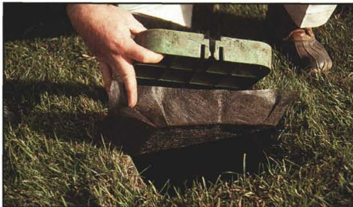
Filter fabric is installed on the lip of the irrigation valve boxes and folded upward around the lid to prevent sediments from entering the submerged valve box.
