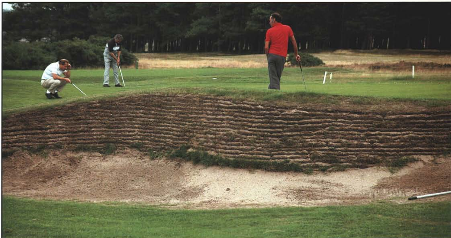
Revetted bunker faces are constructed by stacking thick pieces of sod. The life expectancy of turfed bunker faces depends greatly on orientation to the sun.
