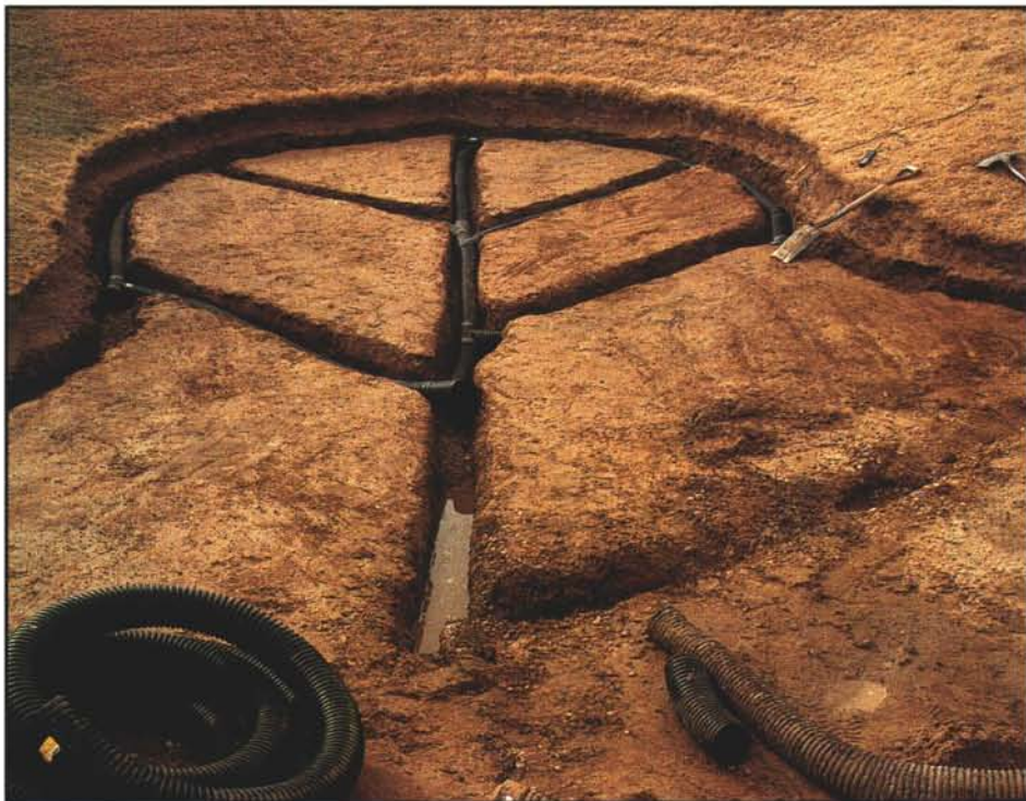
Installing a perimeter drain line under the edge of steep bunker faces can prevent erosion. During a heavy rain the extra drain line captures water from surrounding turf areas and prevents the sand from becoming saturated.
