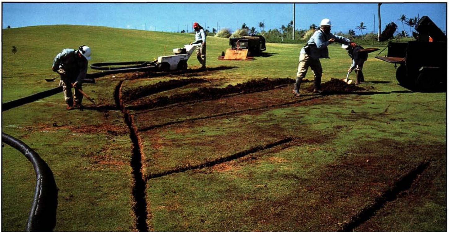
Before considering a fairway topdressing program, make sure your drainage is adequate!
