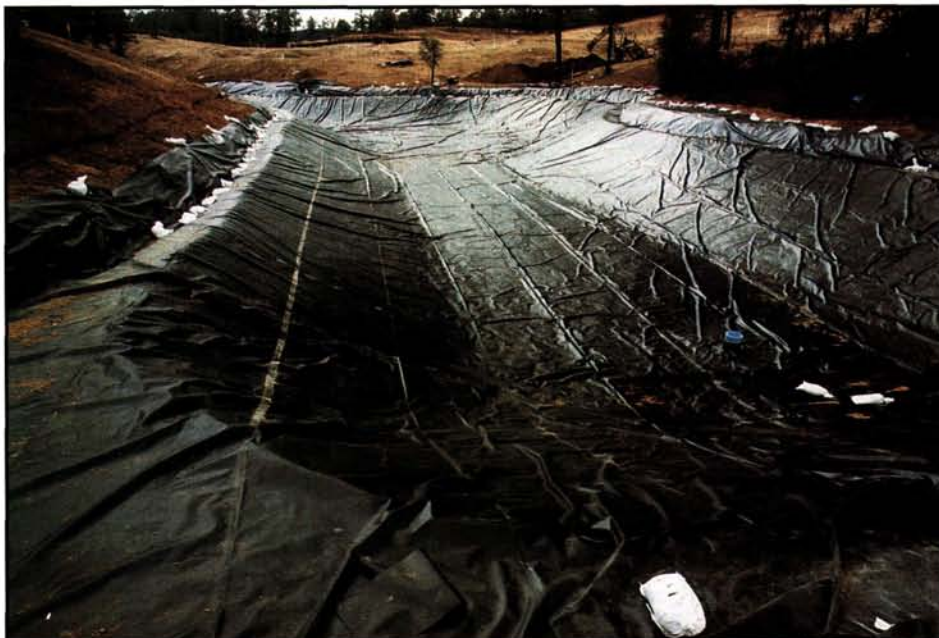
The liner has been spread evenly across the surface. Notice the edge preparation, which ensures a good seal at maximum lake level. The footer at the top has been prepared for the installation of a concrete edge.
