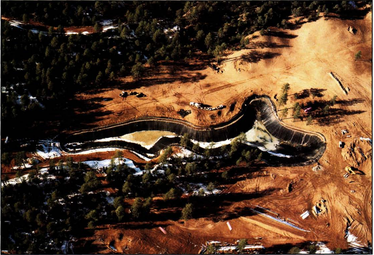
This aerial photo illustrates that even large, variably shaped lakes can be successfully lined when the right materials and proper expertise are employed.
