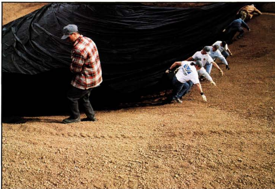
A great deal of manpower is required to pull the liner into place. Also notice how well the lake's bottom is prepared. The surface is compacted, smooth, and free of large sticks and rocks that could puncture the liner.
