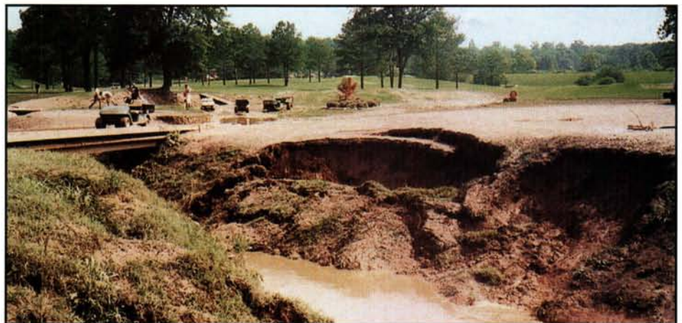
Rapidly flowing water can erode stream banks, which can be prohibitively expensive to repair.
