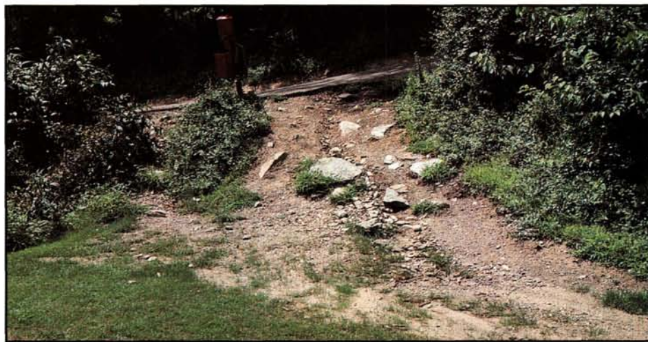
Potential liability situations should be evaluated throughout the golf course. This situation, with golfers exiting the cart path to reach the tee, is an accident waiting to happen.
