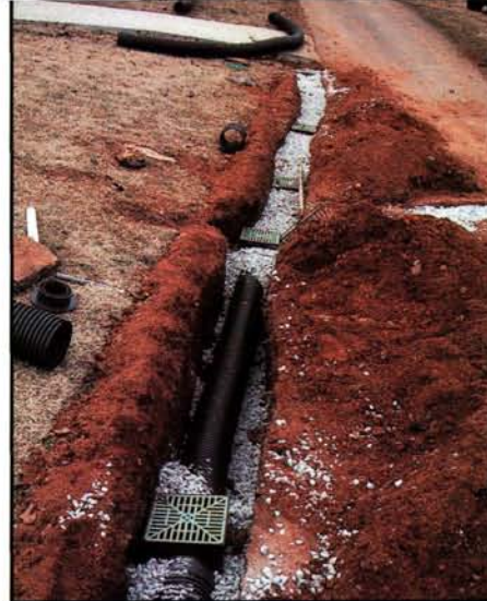
Drainage projects should be clearly marked to alert golfers of a potentially hazardous area.
