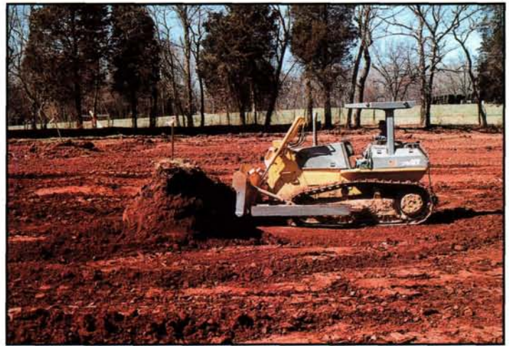
Soil moving is often the most expensive aspect of golf course construction. Deep cuts such as this require the movement of tremendous quantities of soil.
