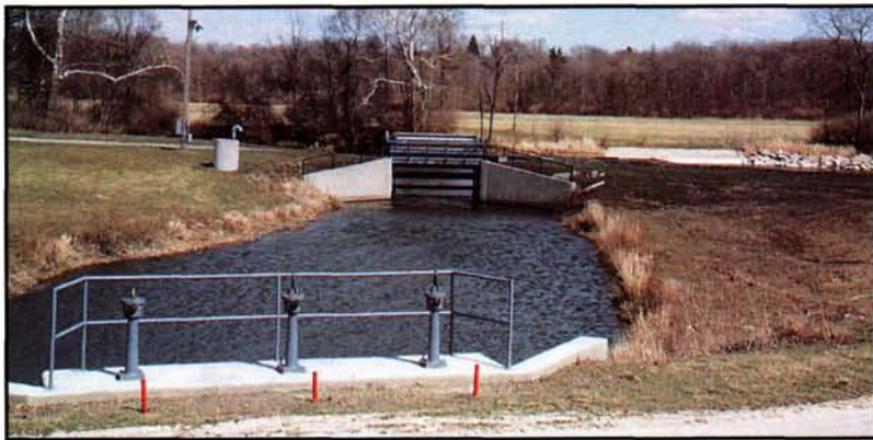
A self-cleaning screen at the lake intake prevents large debris from entering the system.
