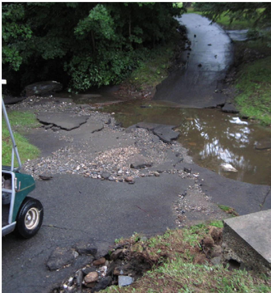
Flooding in late August caused severe damage to cart paths and to the pumphouse.
